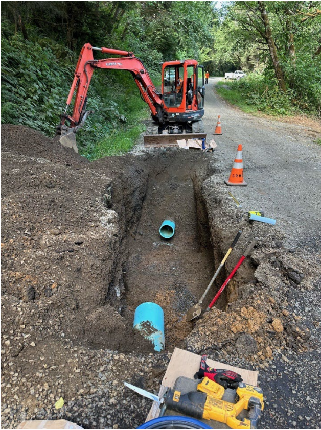
12-inch water mainline settled and offset:
