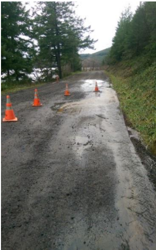
Leaking pipe on 12/18/15:
